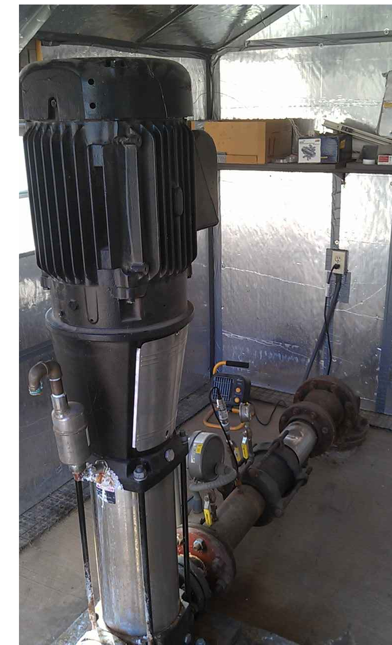
EXISTING PUMP (TO BE RELOCATED)
