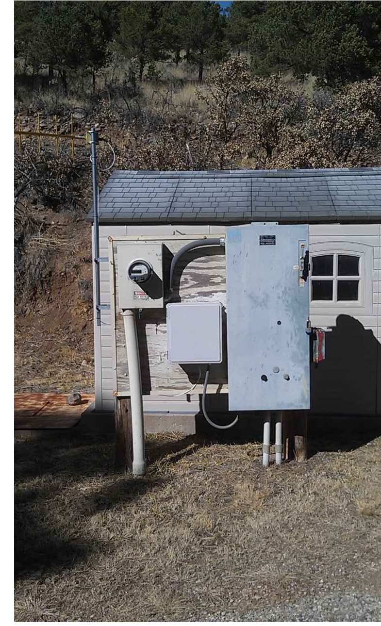
EXISTING ELECTRICAL PANEL (TO BE RELOCATED)
