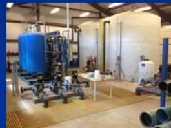
Iron, Manganese Removal and Filtration
